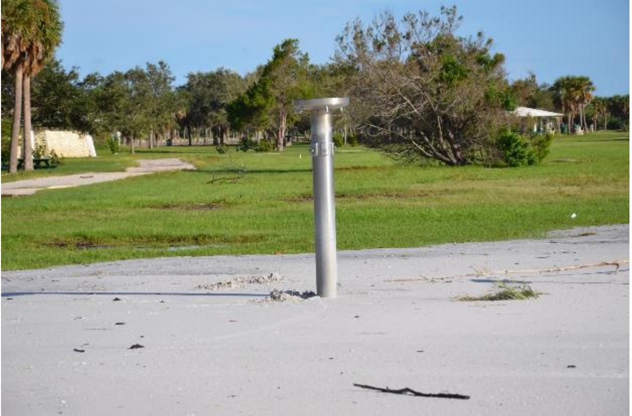
Figure 53. A section of the beach has migrated landward of the previous mangrove swamp. The beach existed before the storm. However, the storm has pushed the beach further landward and partially buried a shower station (lower panel). Note the foot wash faucet is almost at the sand surface.
