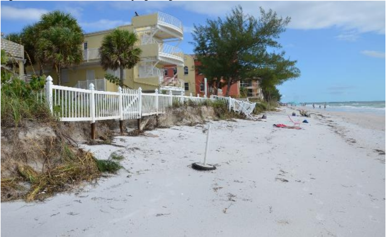
Figure 41. Fence and beach access damage along Sunset Beach.
