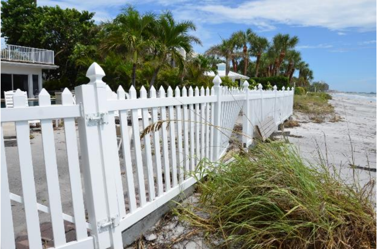
Figure 29. Some structural (fence and beach access stairs) damage with sand washed over the seawall.
