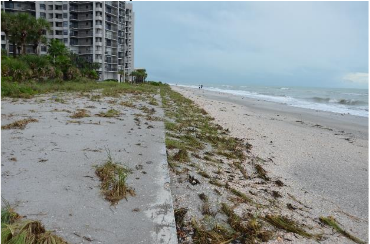
Figure 10. The narrow pre-storm dune was completely eroded, exposing the seawall at the landward limit of the back beach.
