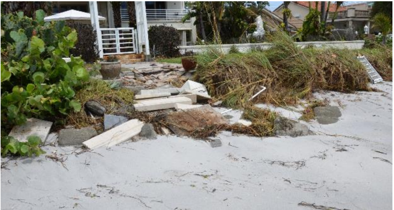
Figure 30. Pavers collapsed due to scour underneath.
