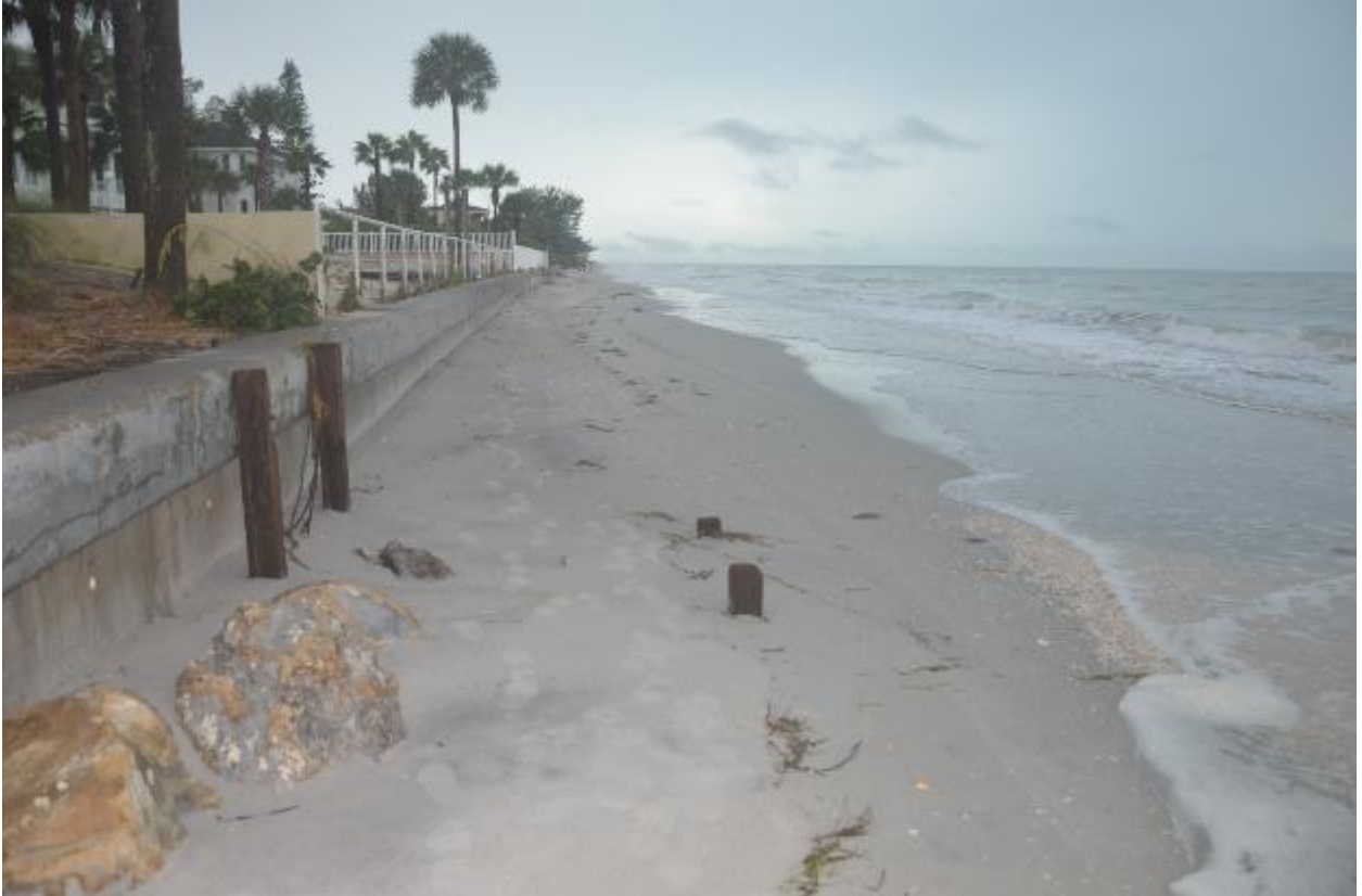
Figure 15. Scour at the seawall, damaging the wood stairs and exposing the riprap.
