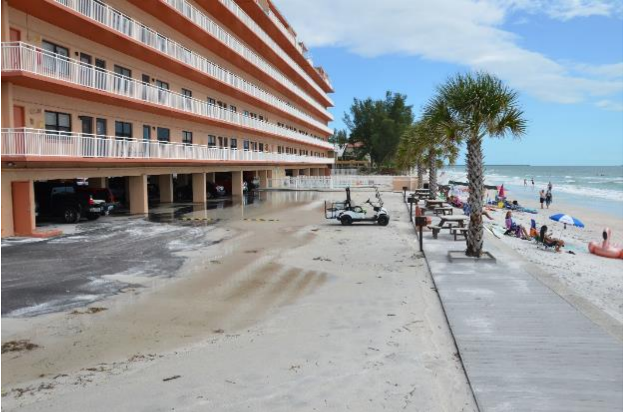
Figure 42. The seawall was overtopped and sand was washed into the parking lot.
