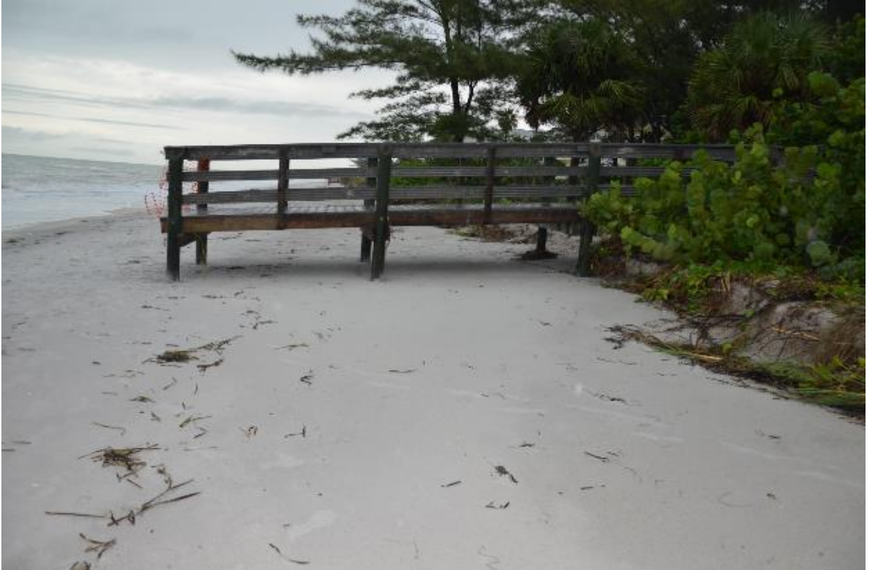
Figure 19. Most of the dune walkovers suffered damage. Upper: dune walkover at Indian Rocks Beach Park, the stairs leading to the beach was washed away. Lower: significant scour underneath and dune erosion of about 10 m (30 ft) at around R72.
