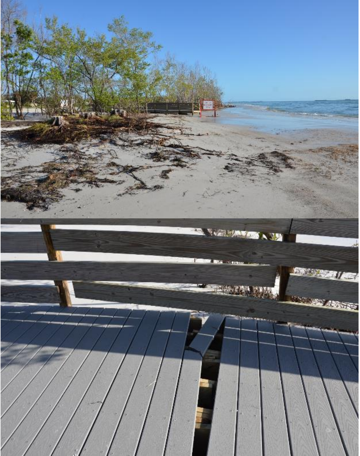
Figure 54. The boardwalk to the beach is severely scoured underneath (upper panel) and was damaged (lower panel).
