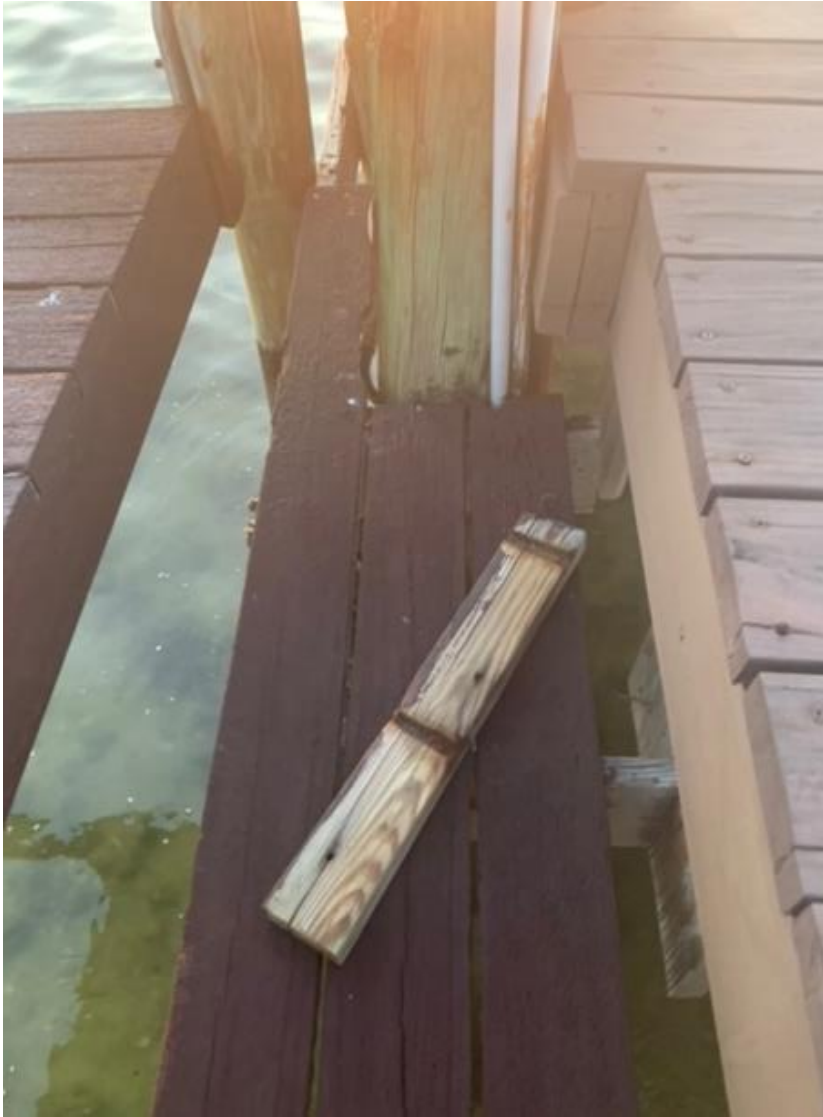
2020 Damage to Dock triggering application for approval
