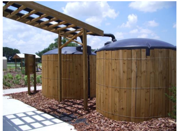
A rainwater harvesting cistern used for irrigation.
