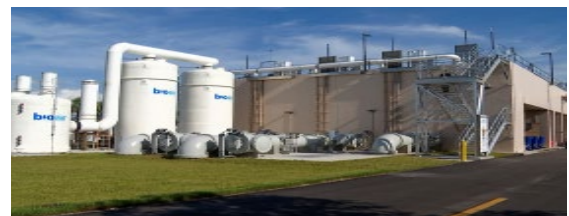
Wastewater treatment plant
