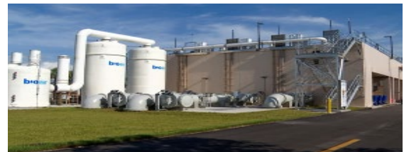
Wastewater treatment plant
