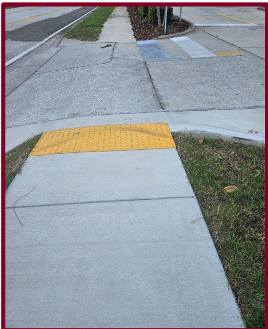
Figure 3 - Detectable warning pad present in one of four required locations
