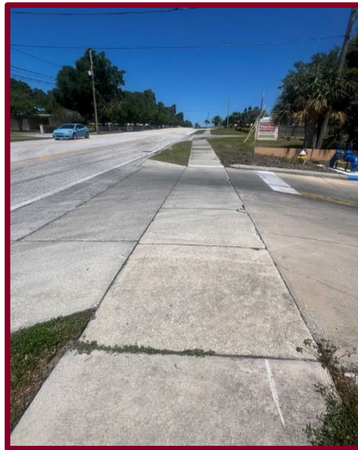
Figure 5 - Detectable warning pads not present in two of four required locations
