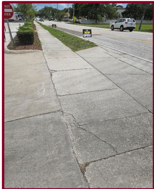
Figure 4 - Detectable warning pads not present in one of four required locations
