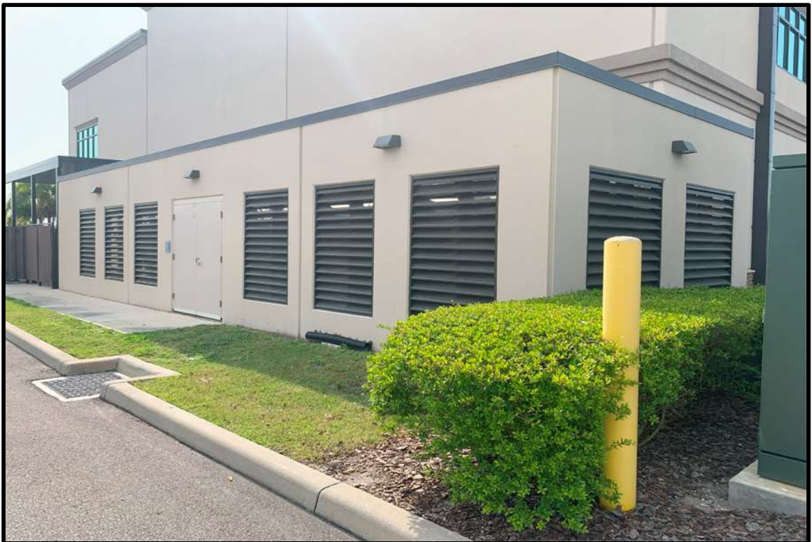
HVAC CHILLER ROOM AT NORTHWEST CORNER OF BUILDING
