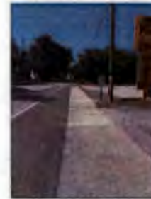
Figure 10: Sidewalk Lacking Separation from the Roadway Source: Kimley-Horn
