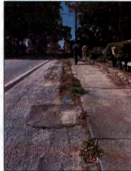
Figure 8: Pavement in Need of Repair on Philippe Parkway Source: Kimley-Horn
