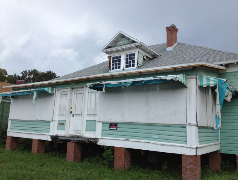
Photo 1a: Pre-rehabilitation frontal elevation, deteriorated clapboard siding/trim, and enclosed porch.
