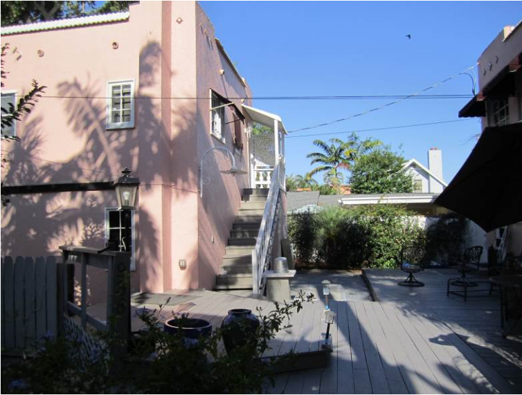
Photo 4a. Pre-rehabilitation garage apartment with deteriorated stair system.
