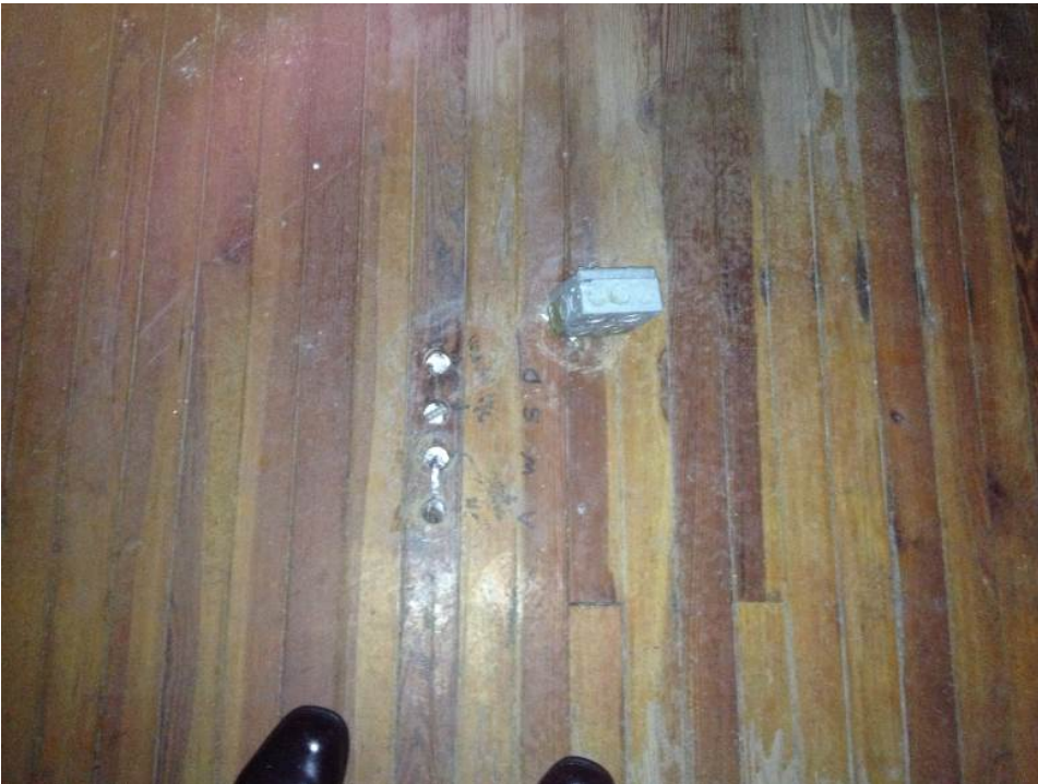
Photo 2a: Pre-rehabilitation wood floor damage (typ.).
