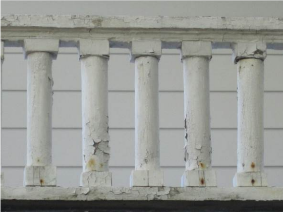
Photo 4a: Balustrade deterioration.
