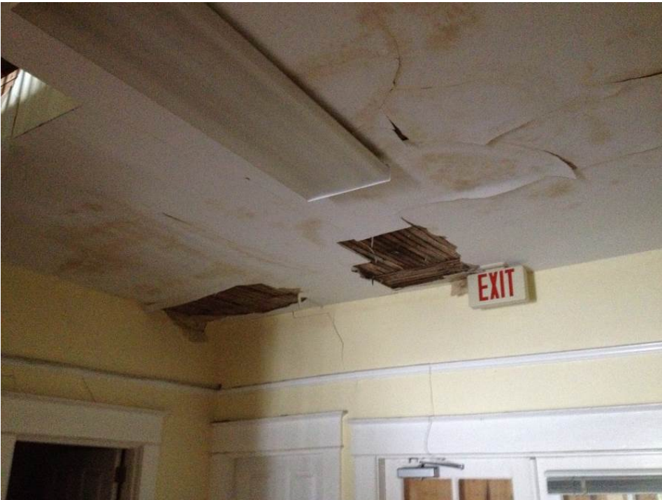
Photo 3a: Pre-rehabilitation interior damage (typ.).
