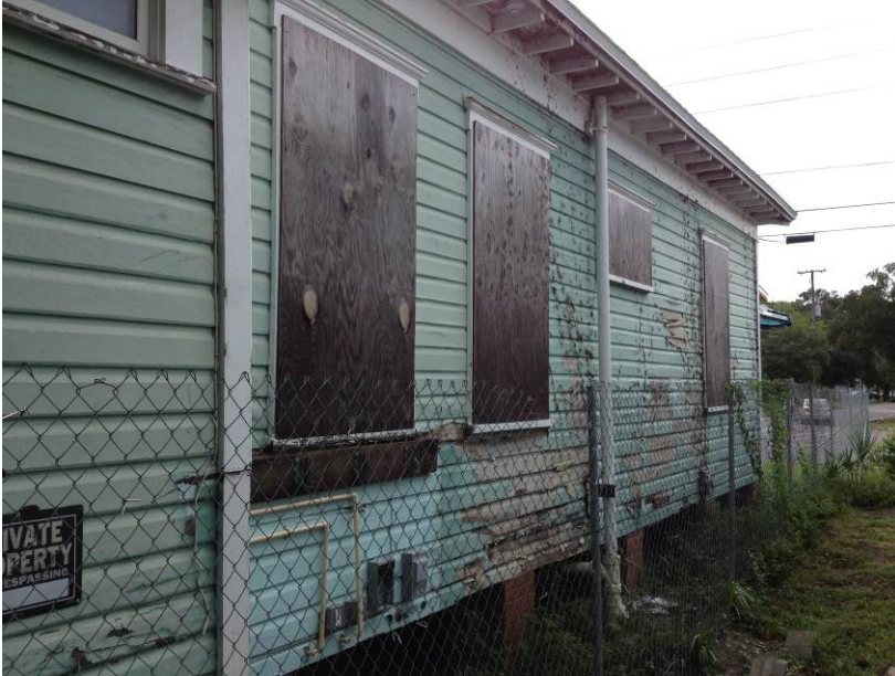
Photo 1c: Pre-rehabilitation side elevation clapboard siding damage and boarded window elements.
