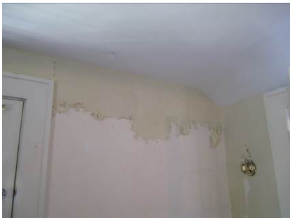
Photo 6a. Wall damage (typ.).
