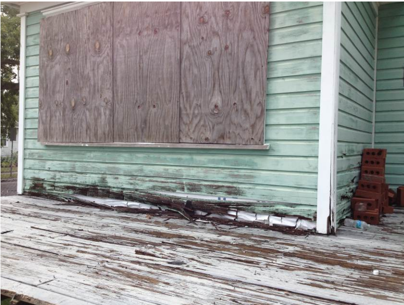
Photo 1b: Pre-rehabilitation deteriorated clapboard siding and non-historic deck attachment.
