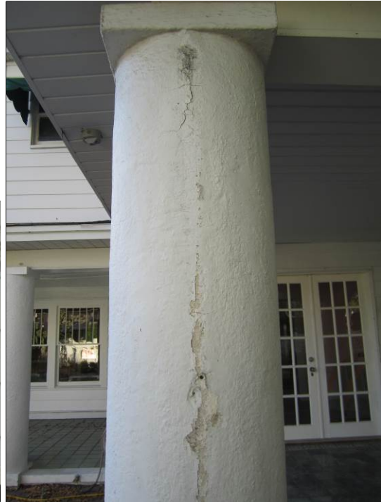
Photo 4b: Column damage.
