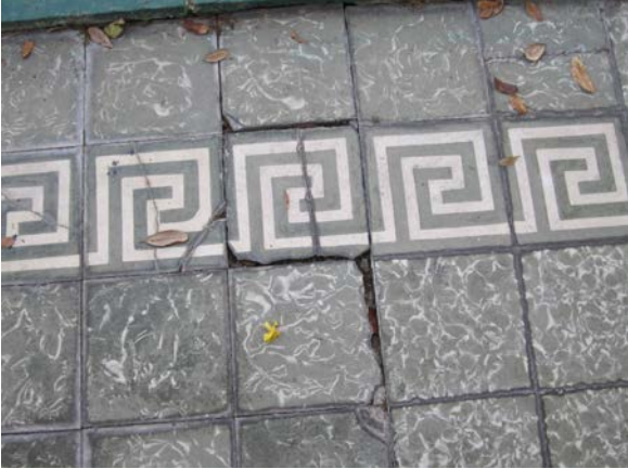
Photo 5a: Damaged porch tile.
