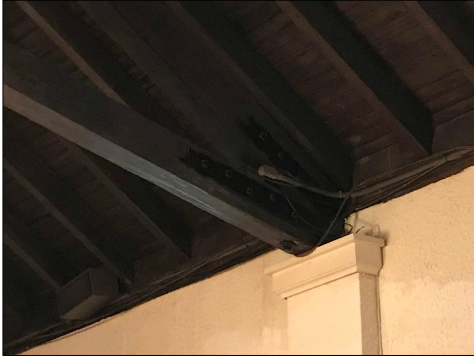
Figure 8: Interior truss and connector
