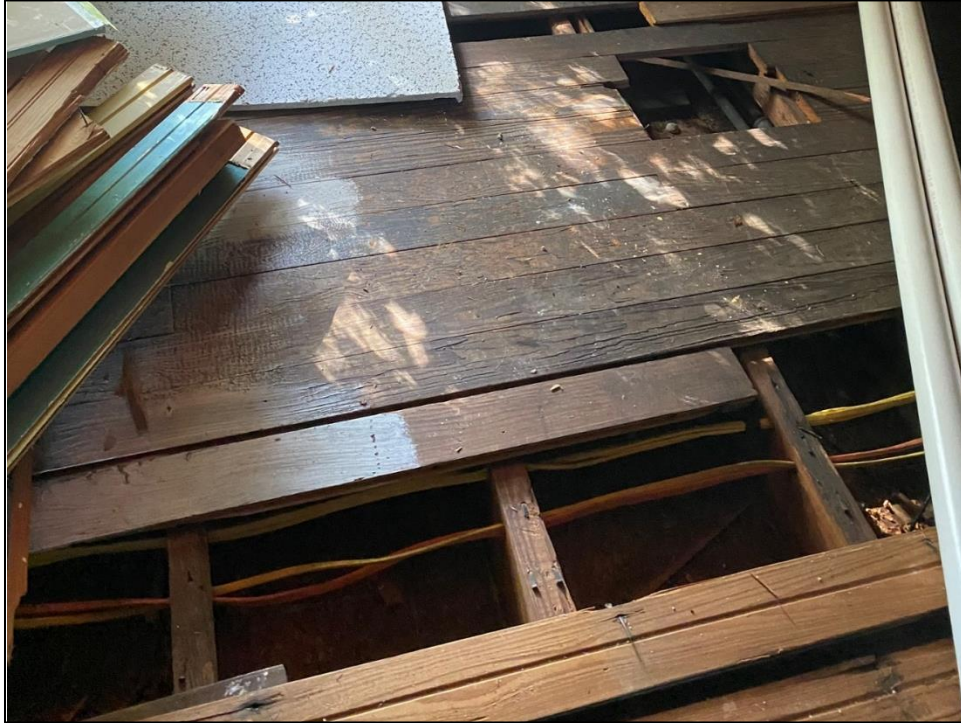
Figure 9: Disused wiring in attic
