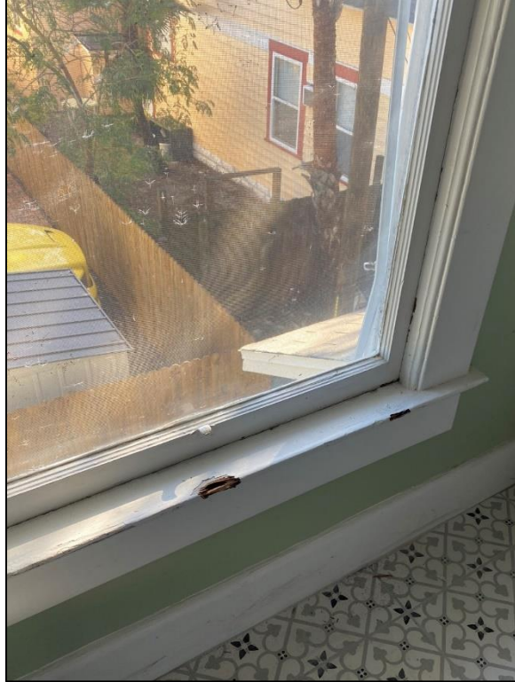
Figure 11: Damaged wood window sill and casings
