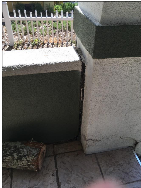
Figure 4: Separation accruing at front porch due to tree roots
