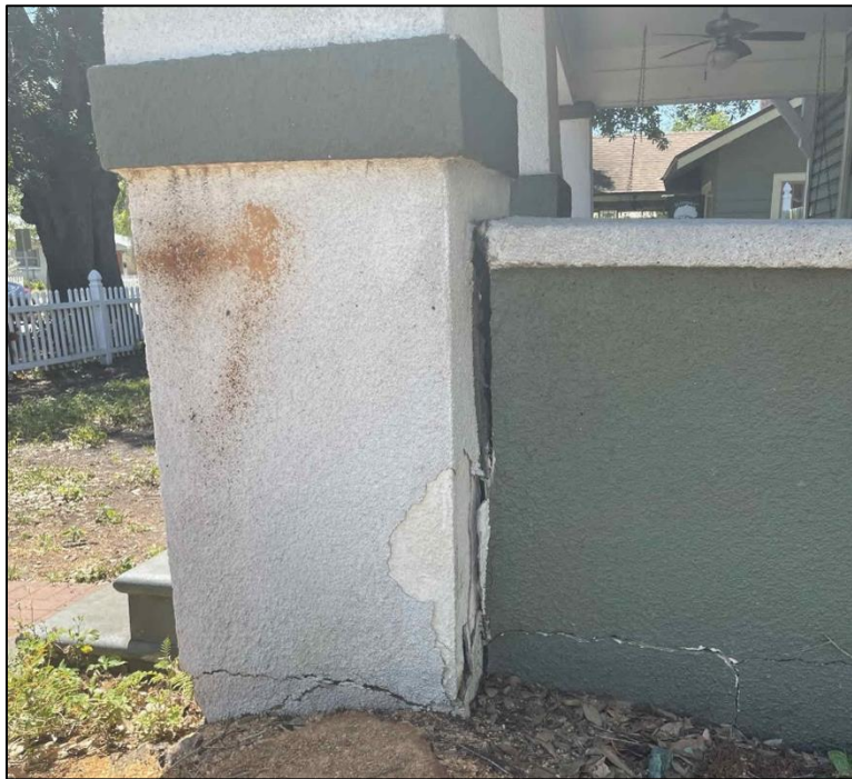
Figure 6: Another detail of porch damage from tree
