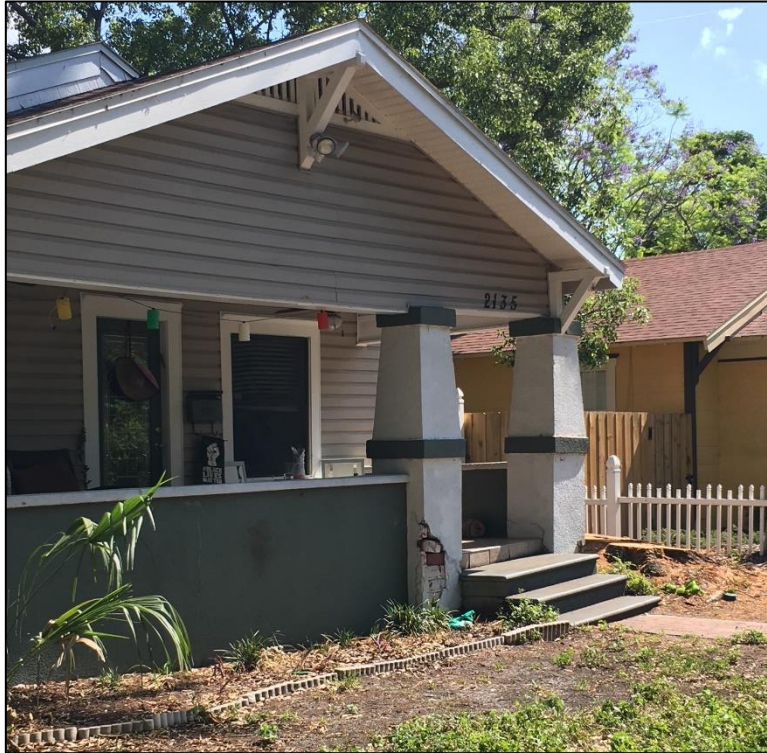
Figure 3: Damage can be seen at porch columns
