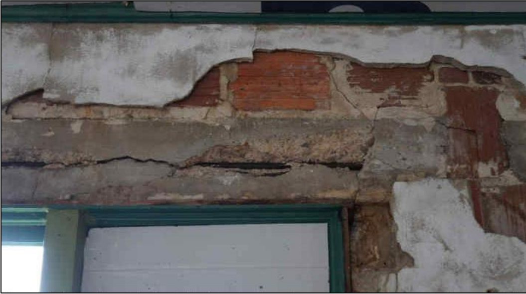
Figure 7: Deteriorated concrete lintels
