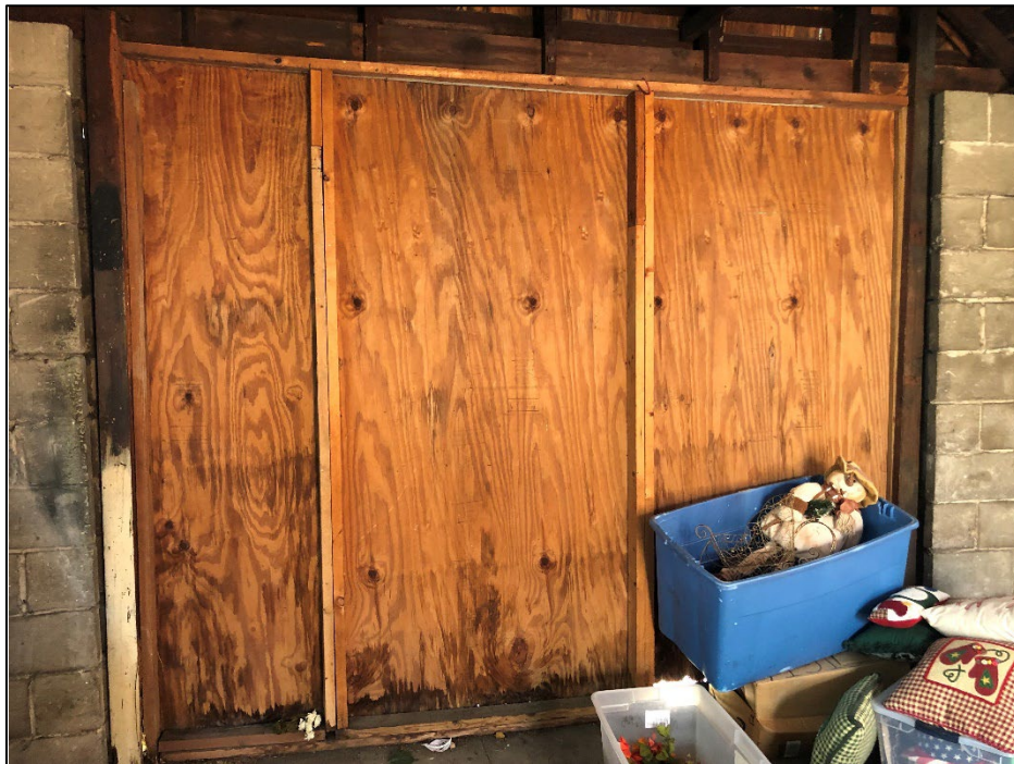
Figure 6: Rear wall with rotted wood
