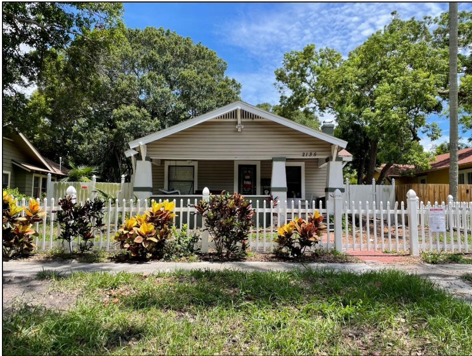
Figure 2: Front façade after tree removal, and damage apparent from tree. See leaning right column.
