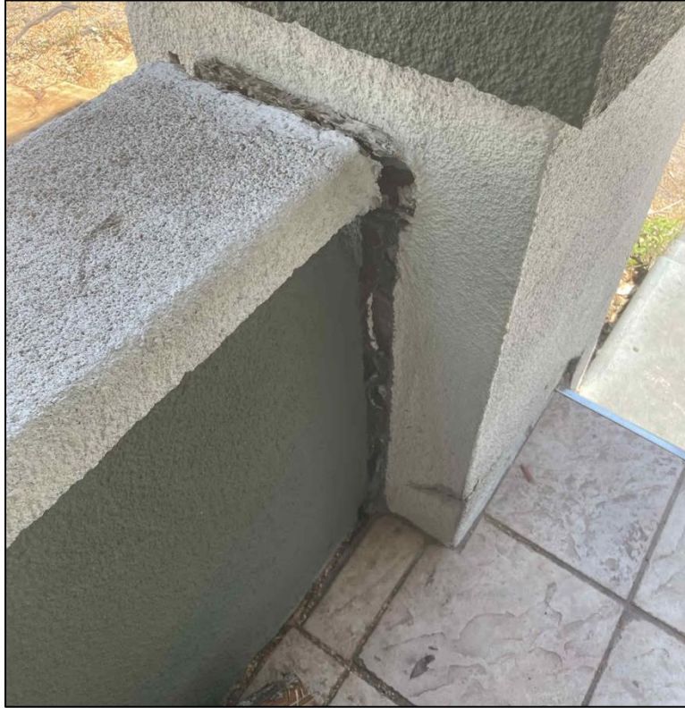
Figure 5: Detail photo of porch separation
