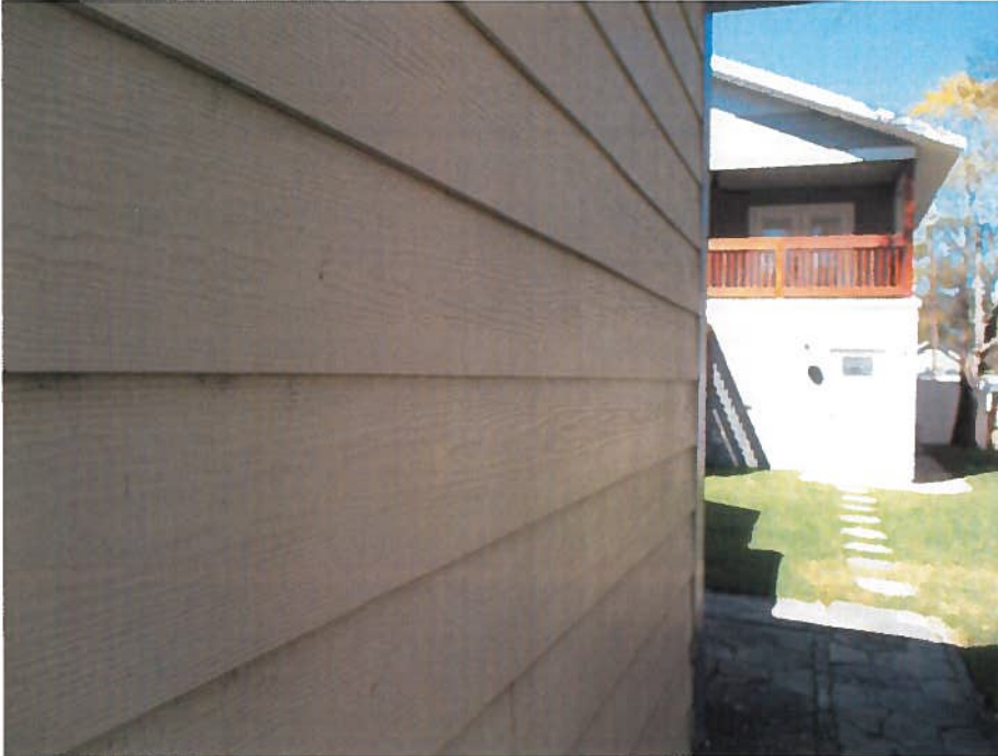
Photo 3: HardieBoard exterior siding on main contributing house was matched at new construction shown to rear. Photo by Staff, 2018.
