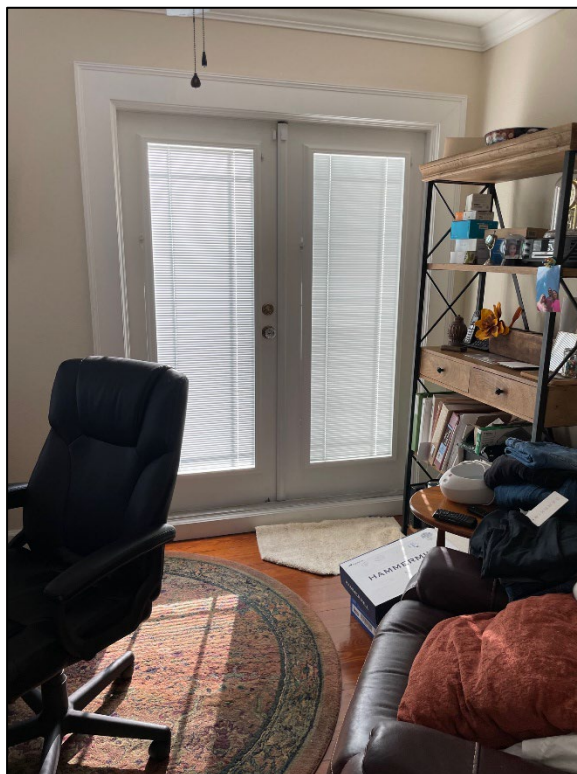
Figure 13: French doors to be replaced, prior to construction
