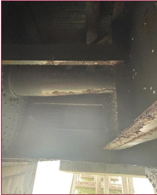
Figure 7 - Structural Steel Framing Beneath the Dunedin Causeway Bridge Showing Heavy Rust Buildup
