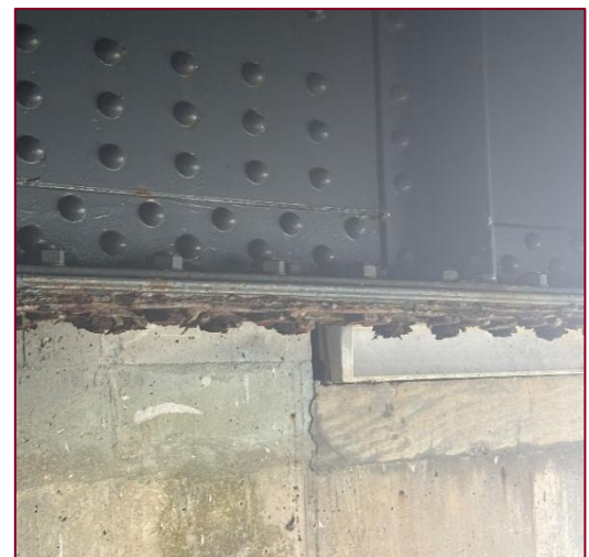
Figure 6 - Close-up View of Heavy Rust Buildup on the Underside of the Dunedin Causeway Bridge
