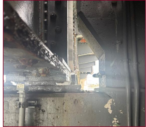
Figure 8 - Additional Underside View of the Dunedin Causeway Bridge Showing Heavy Rust Buildup
