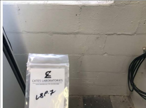
Photo #13 Vault – Interior – West Room – South Wall – Concrete Masonry Unit Walls – Sample Location ( LBP-7 )
