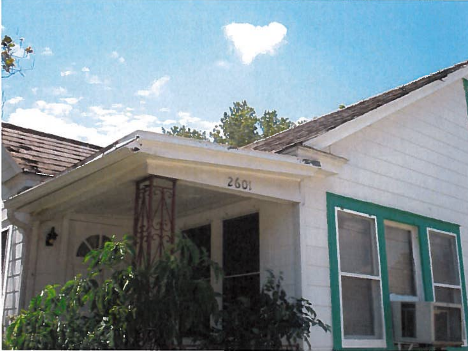
Photo 1: Asbestos roof deterioration. Photo by Staff, 2016.
