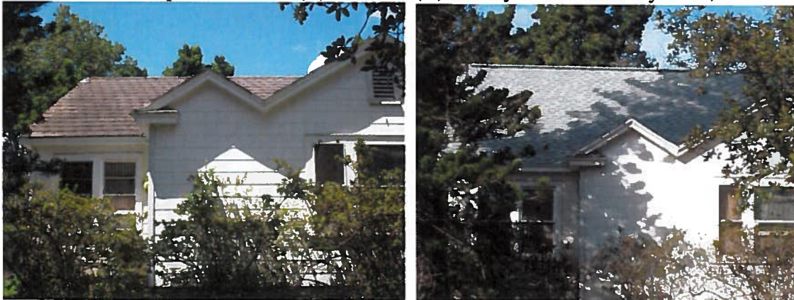
Photos 4, 5: Comparison of old (L) and new (R) roof systems. Photo by Staff, 2017.
