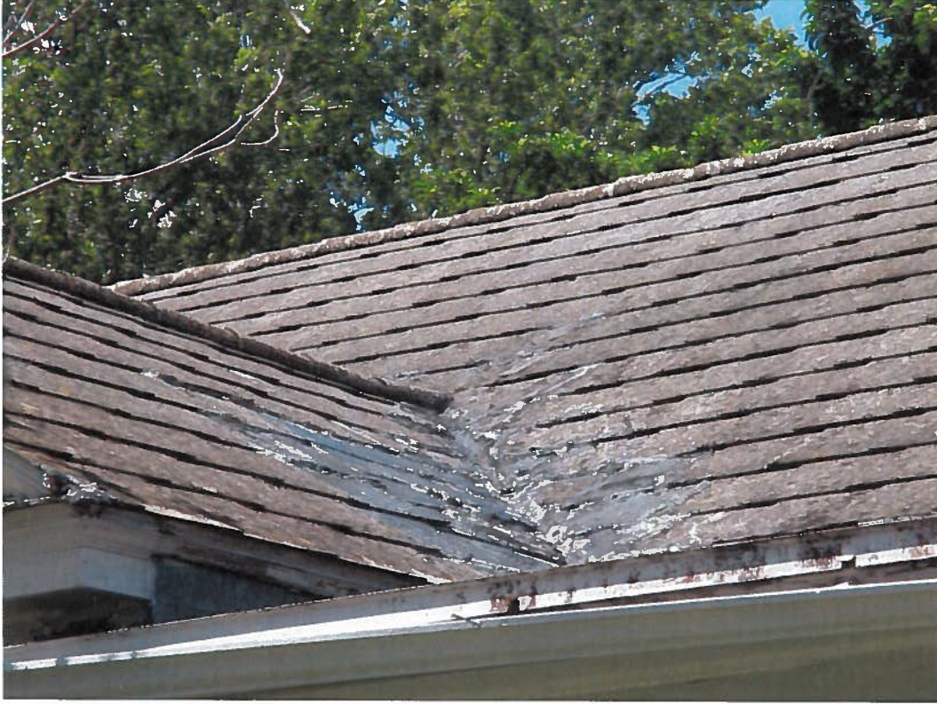
Photo 3: Roof shingle damage at valley (typ.). Photo by Staff, 2016.
