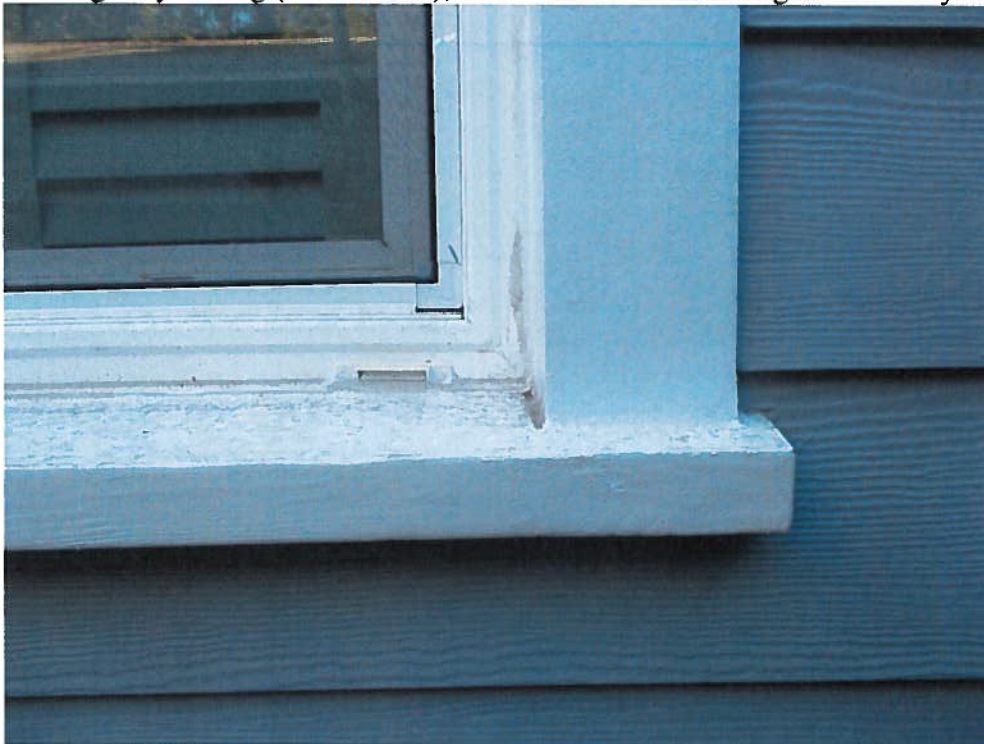
Photo 7: New Hardie board siding reveals a more appropriate treatment versus the pre-existing vinyl siding (see Photo 6), and earlier asbestos shingles. Photo by Staff, 2017.
