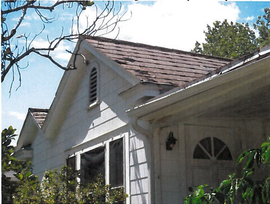
Photo 2: Deteriorated asbestos shingles-front entry. Photo by Staff, 2016.
