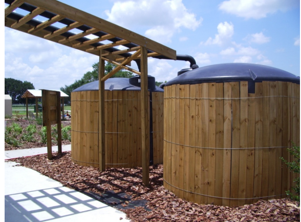
A rainwater harvesting cistern used for irrigation.
