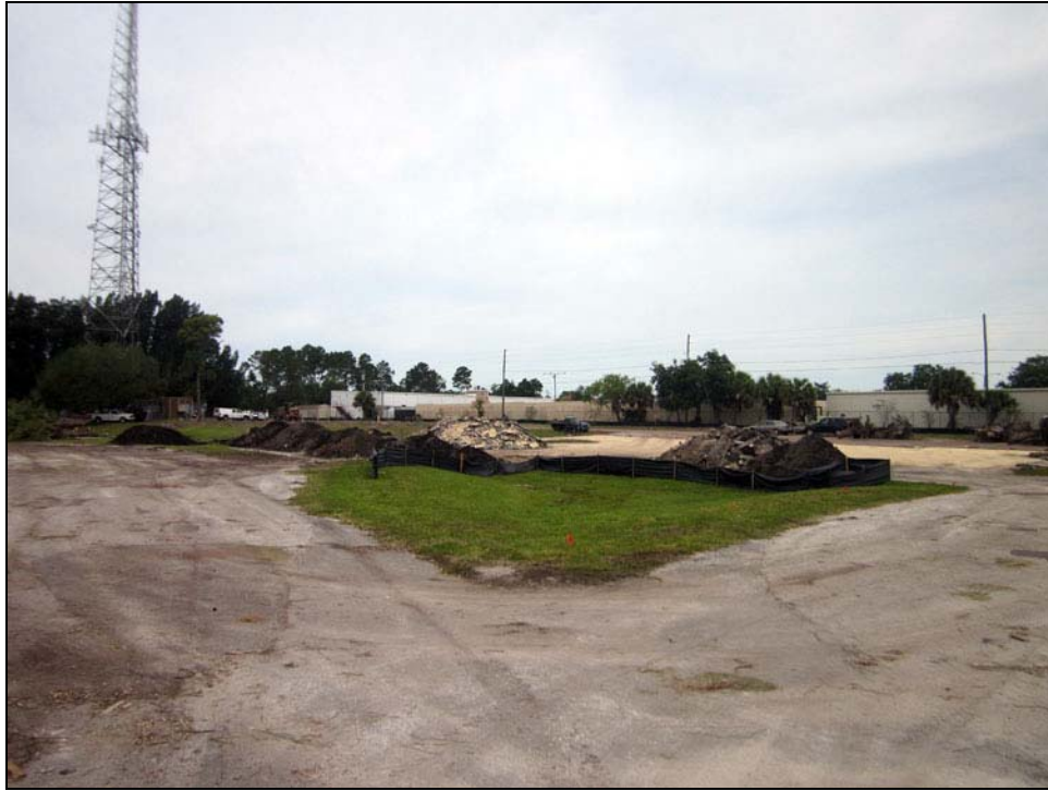
Photo 11: View looking NW at westerly portion of the site showing site work underway. (Taken 4/25/2019)
