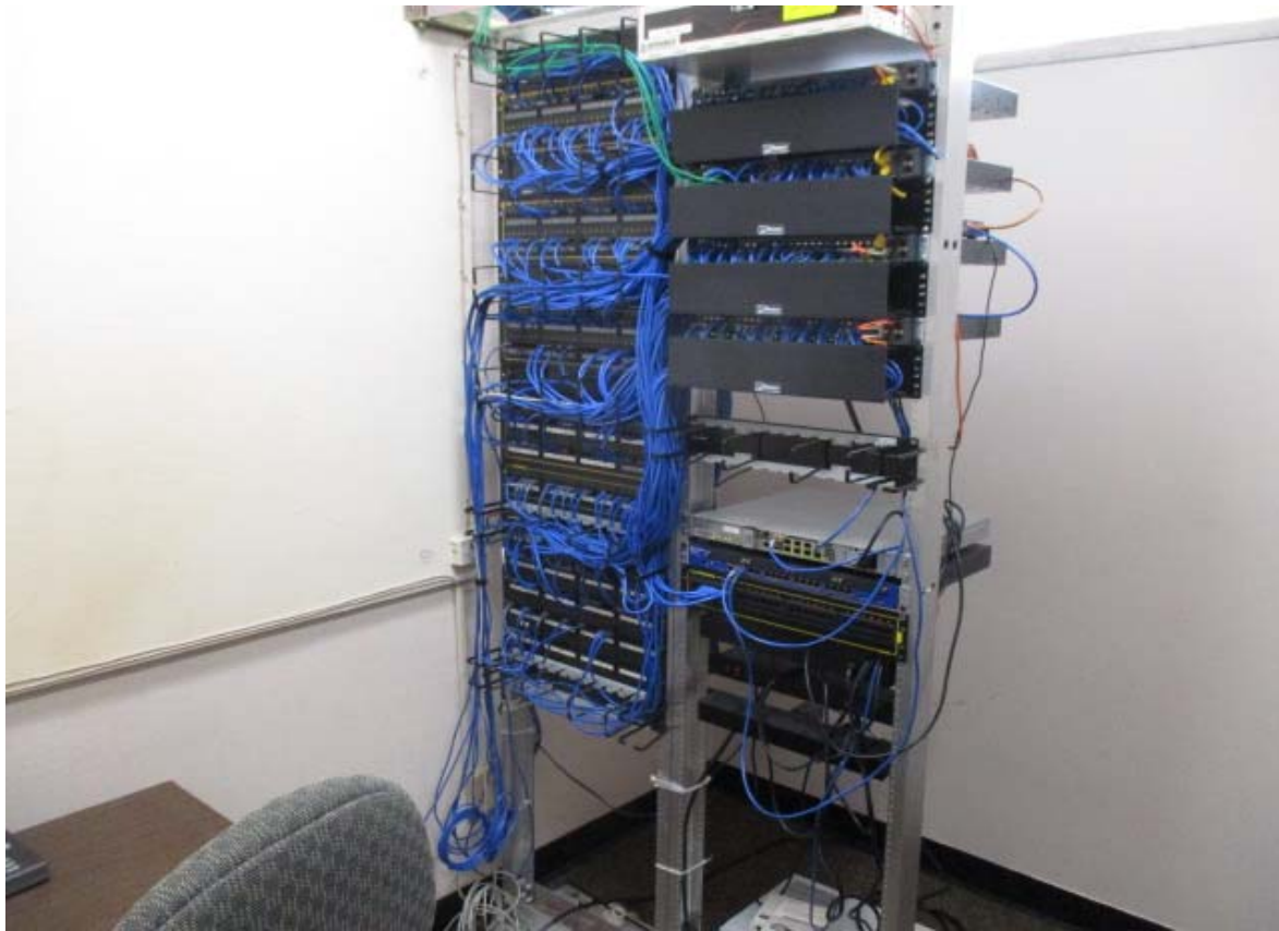
CAT NETWORK WIRING
