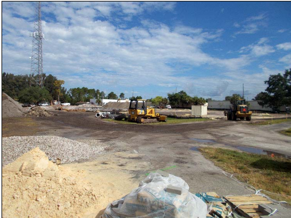
Photo 12: View looking NW at westerly portion of the site showing on-going redevelopment (Taken 6/7/2019).
