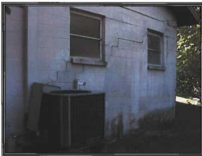
Northwest Corner of the Fellowship Hall/Office Showing the Settlement Cracking
