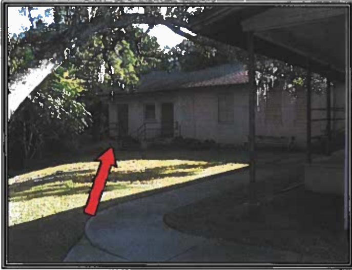
Northwesterly Sides of the Fellowship Hall/Office Red Arrow Indicates Corner of Building Where There are Settlement Issues
