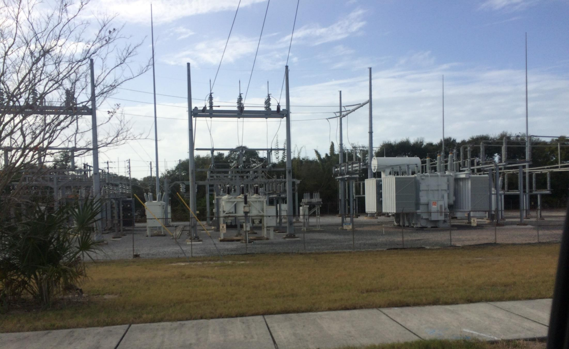
Power substation (across Tampa Rd.)
