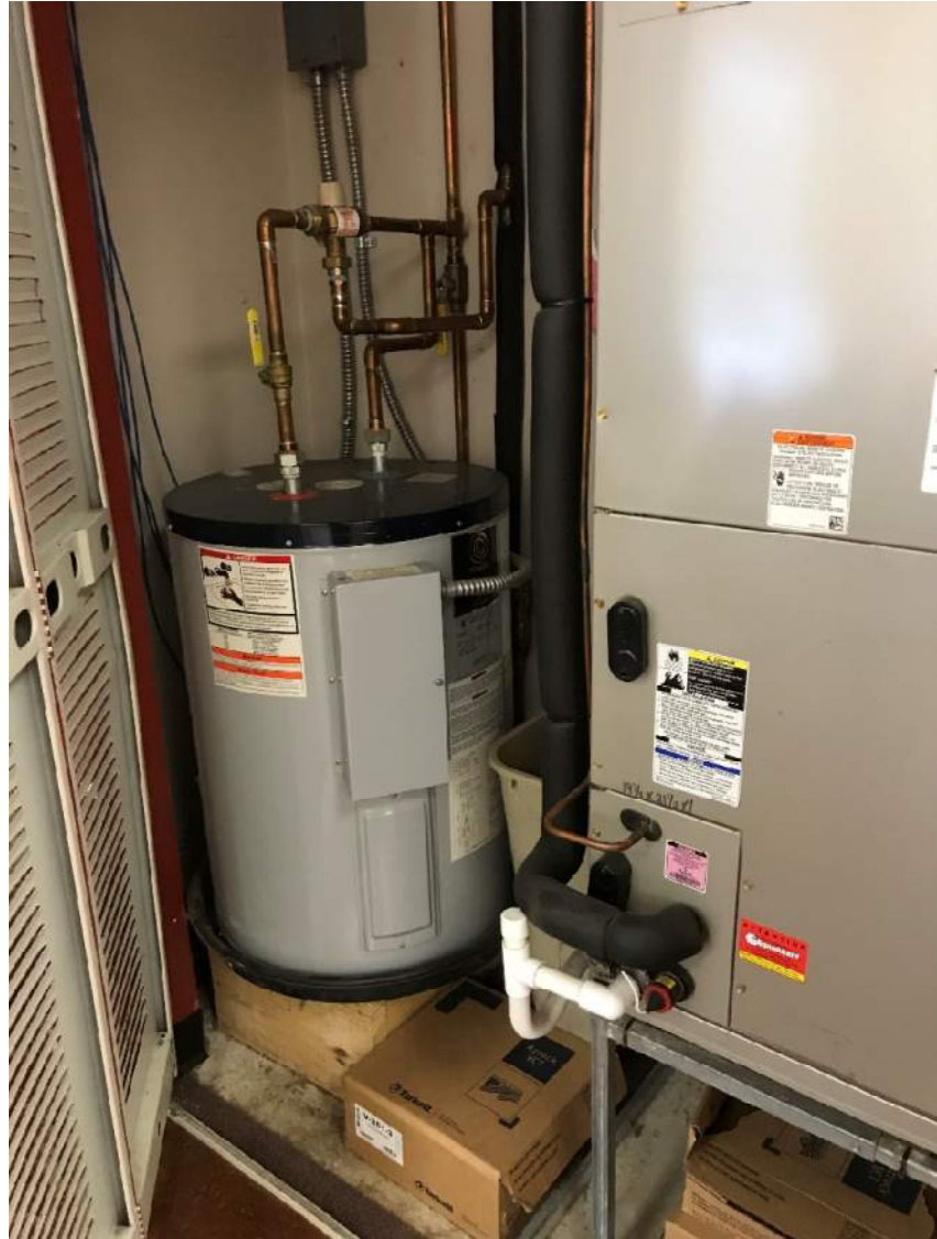
GYM WATER HEATER
