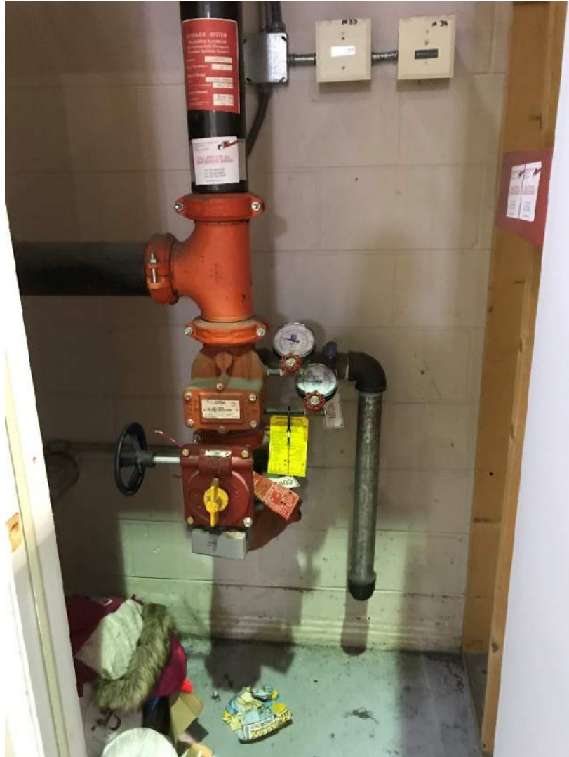
GYM SPRINKLER RISER
