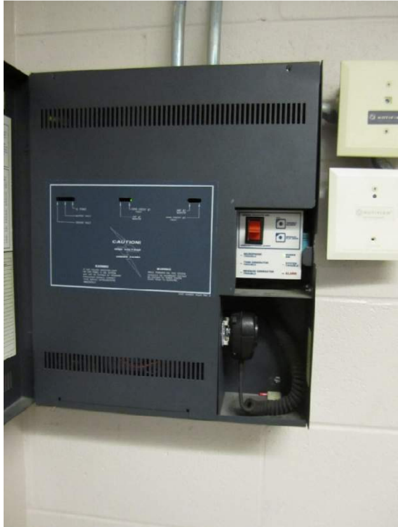
GYM FIRE ALARM
