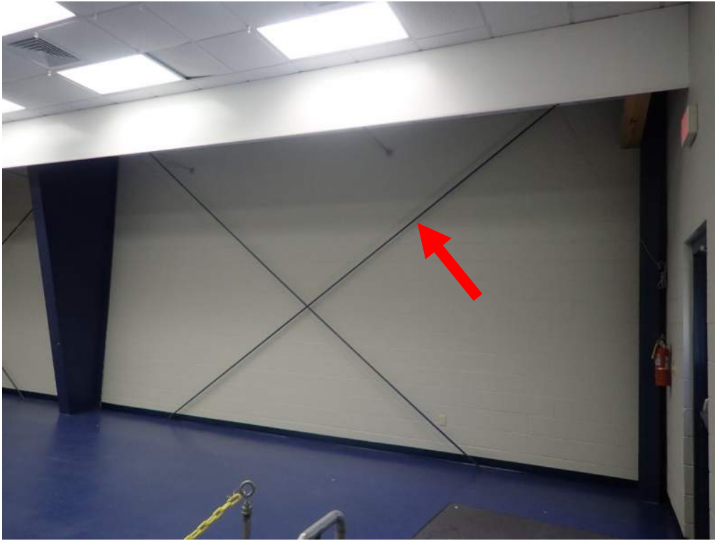
Photograph 7 – Loose X bracing in Rigid Frames
