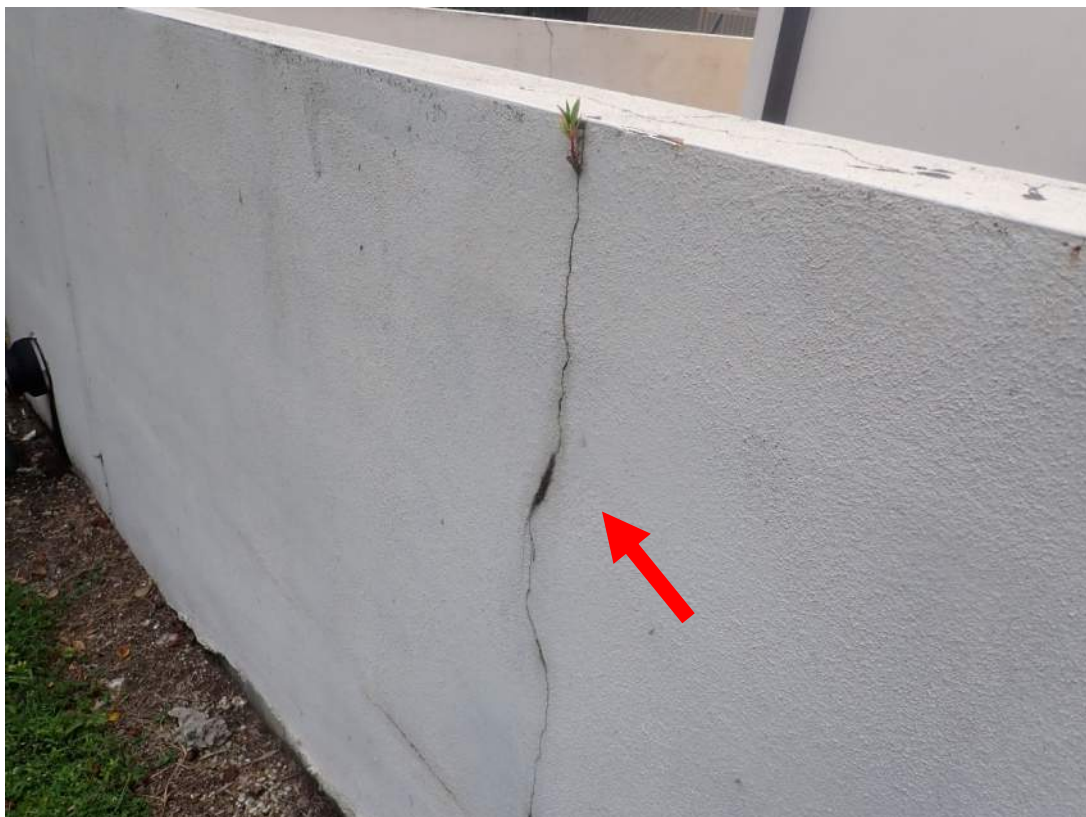
Photograph 12 – Cracks In Site Wall At South East Corner
