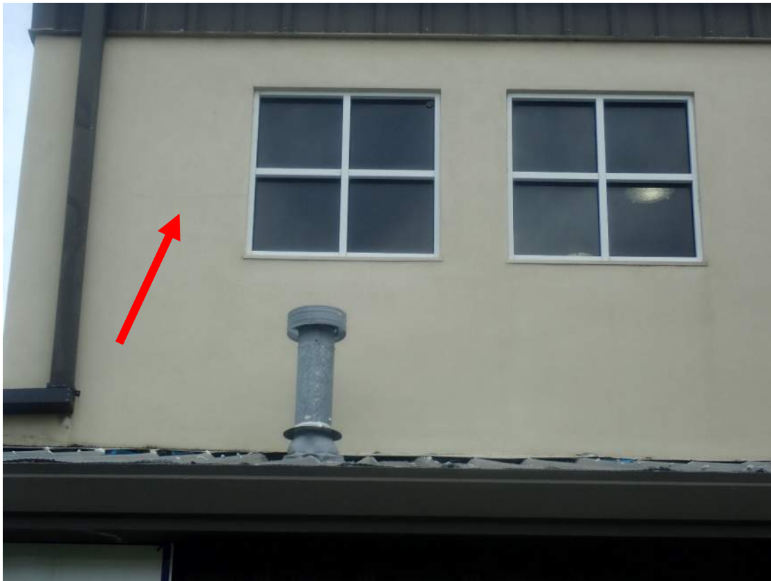
Photograph 15 – Example of Stucco Cracks Near Windows In Exterior Walls of Gym
