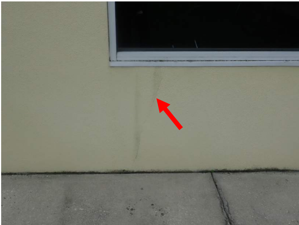
Photograph 14 – Example of Stucco Cracks Near Windows In Exterior Walls of Gym
