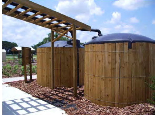
A rainwater harvesting cistern used for irrigation.
