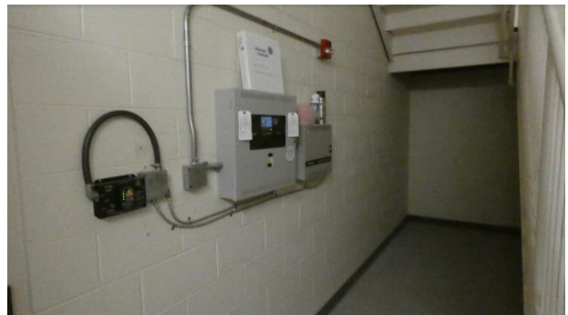
16. Bldg. A fire system control
