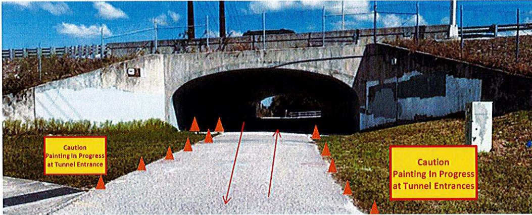
Tarpon Springs WEST CONE LAYOUT for Artists Painting Sides of Tunnel Face
