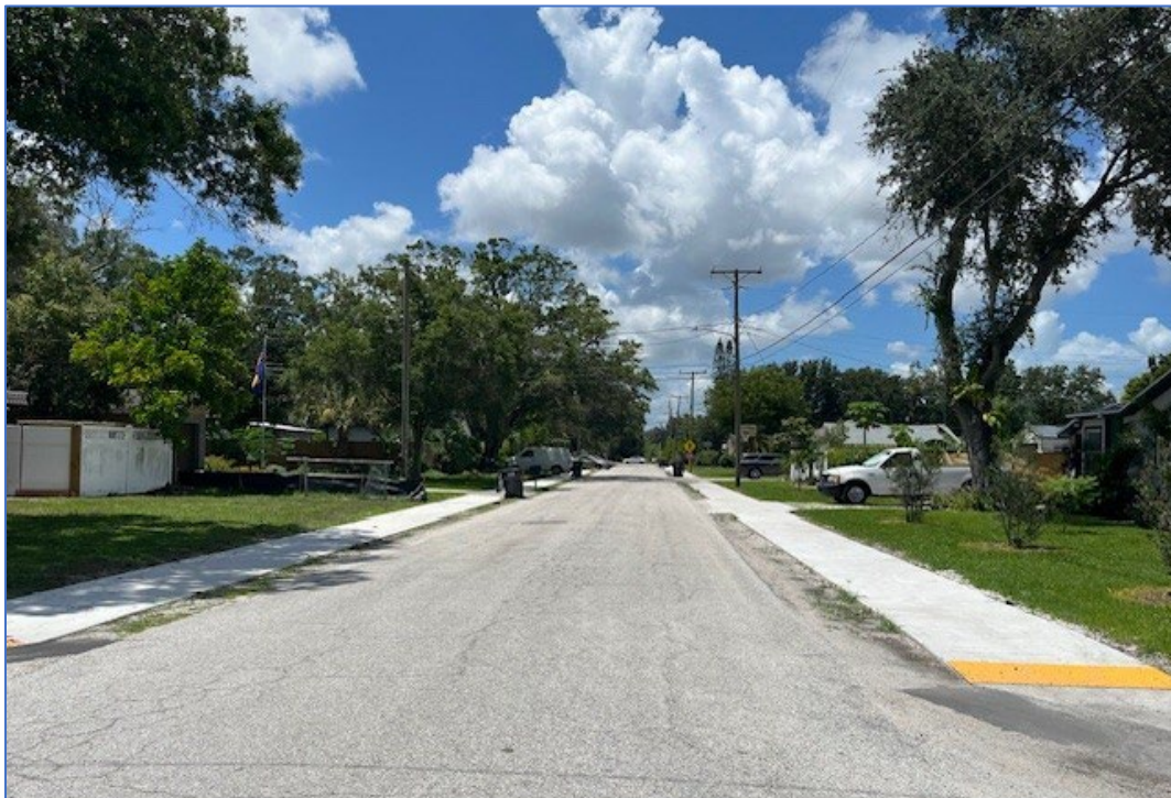
39th St. N. sidewalk constructed connecting the Neri Park and the Lealman Elementary School
