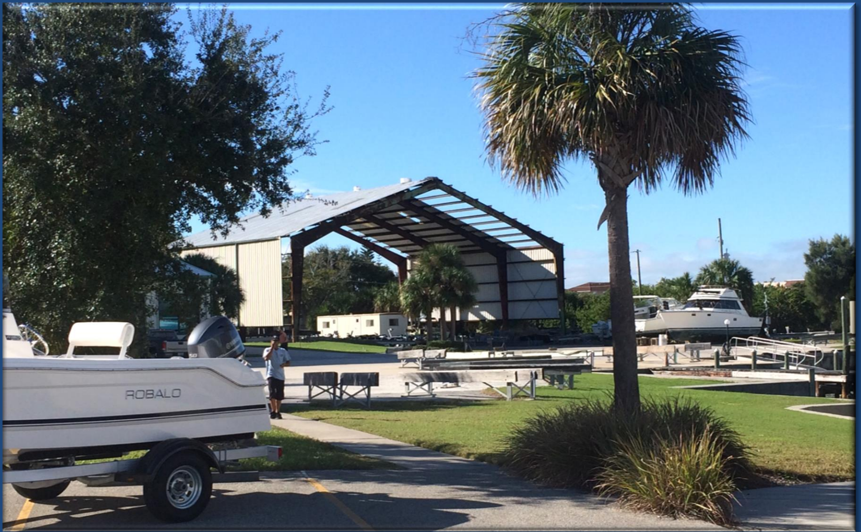
Inside marina – storm damaged building
