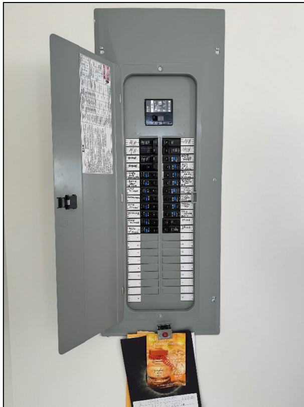
Figure 22: New electrical panel, post construction
