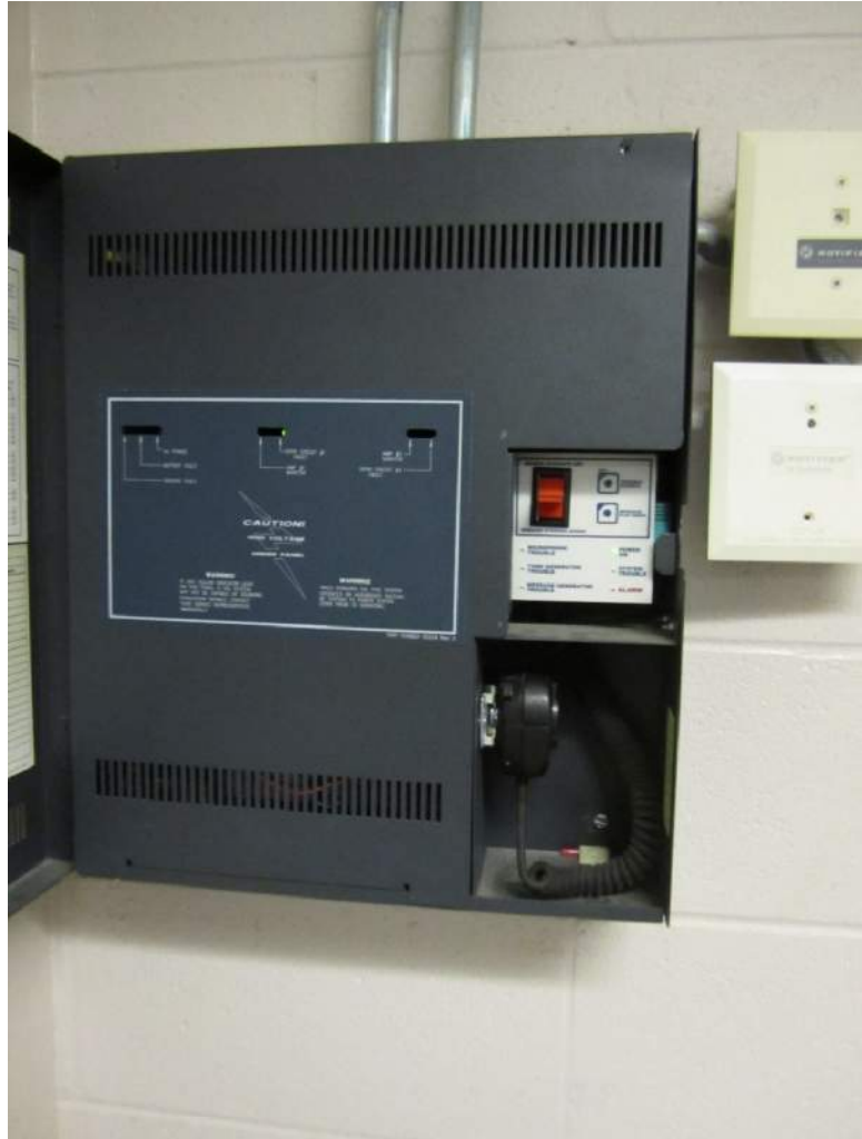
GYM FIRE ALARM
