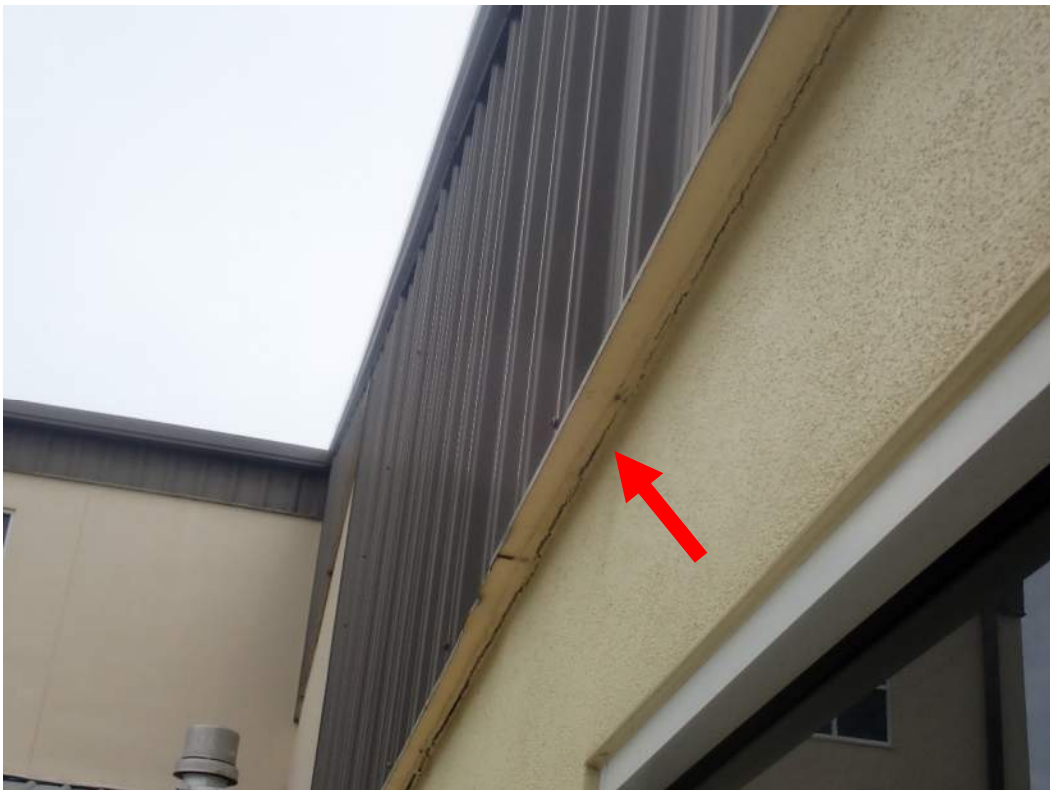
Photograph 10 – Damage and Separation at Metal Wall Flashing
