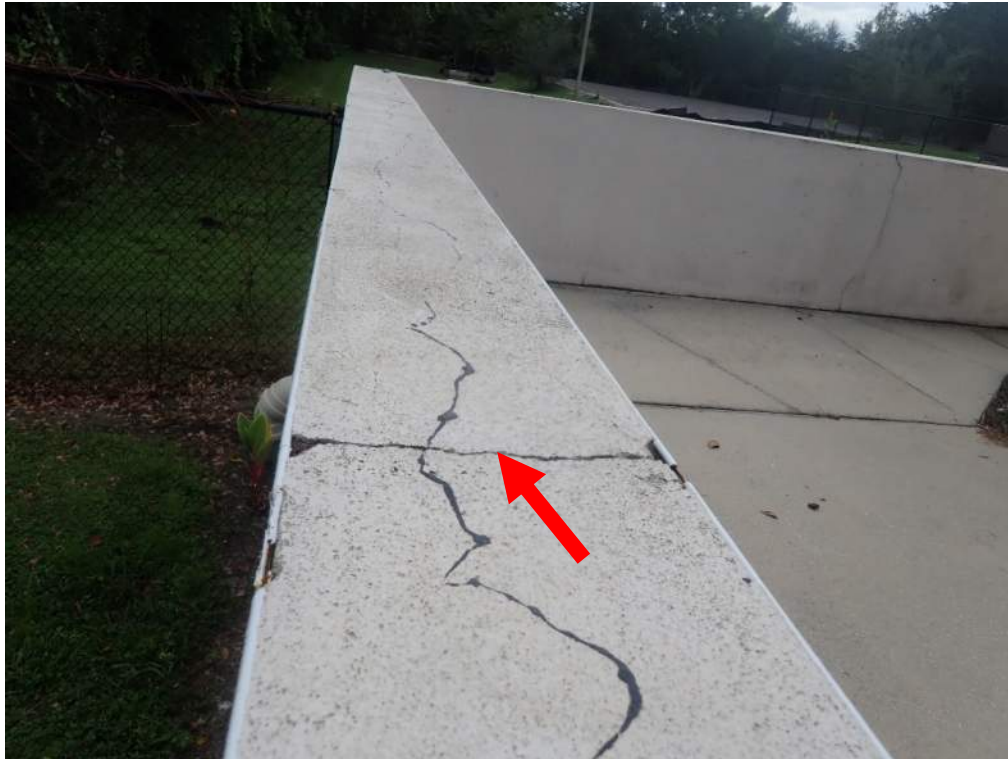
Photograph 13 –Cracks In Site Wall At South East Corner
