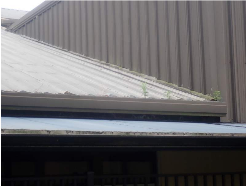
Photograph 9 – Vegetation Growth at Roof Edges
