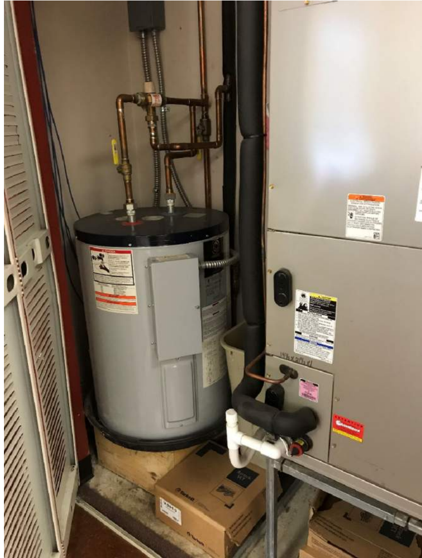
GYM WATER HEATER
