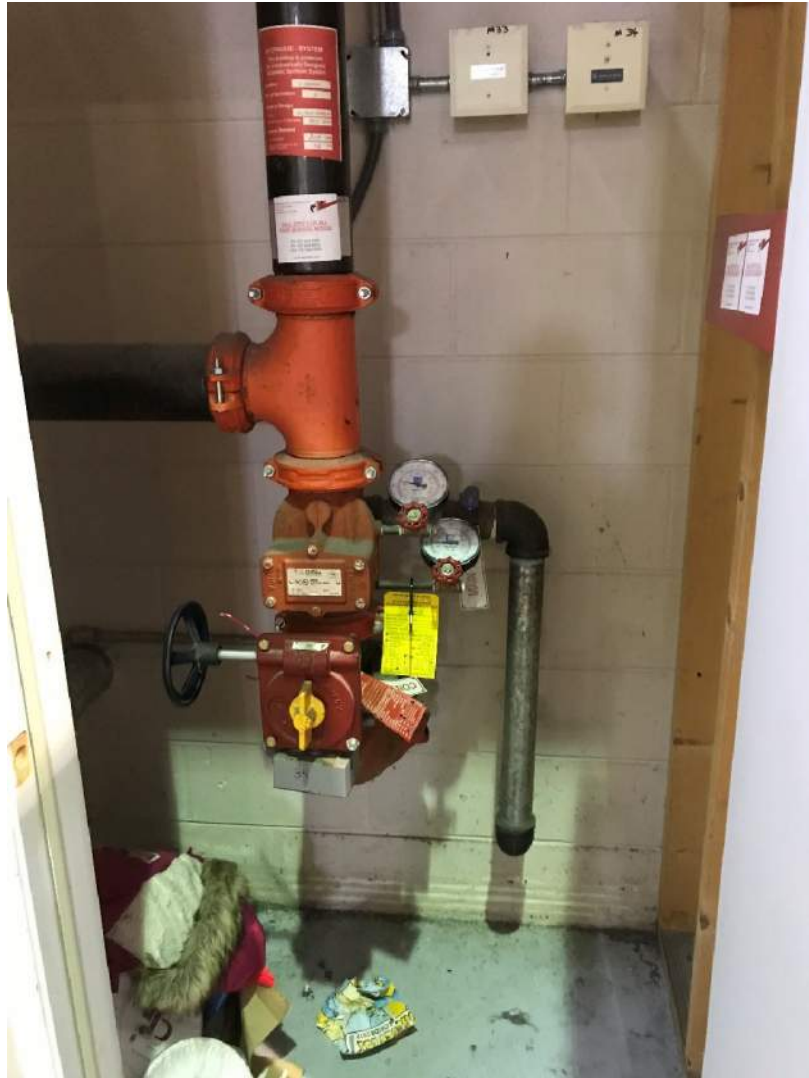
GYM SPRINKLER RISER
